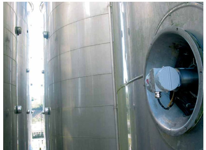
Figure 4: DT302S Installed on a Fermentation Tank
