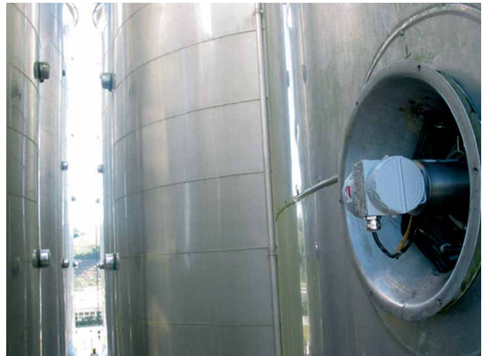
Figure 4: DT302S Installed on a Fermentation Tank
