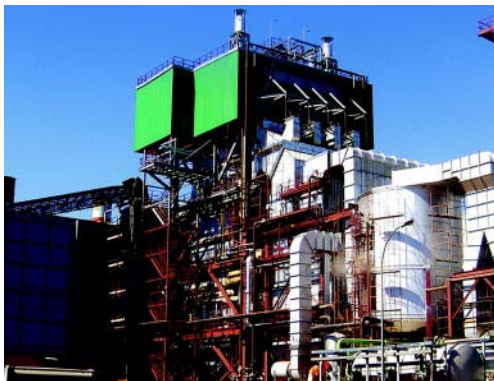
The new thermoelectric power plant
