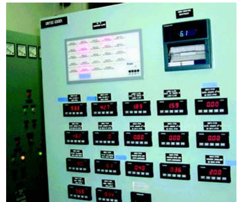
Painel de controle
