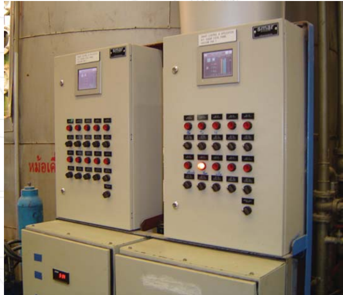
Details of Local Control Panel (see HIM detail)
