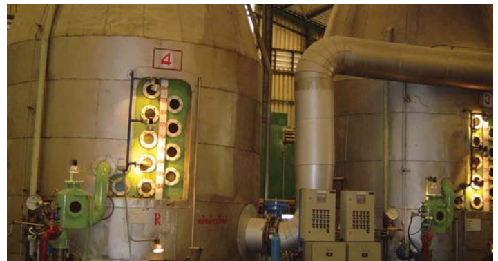
Refined Vacuum Pans Area
