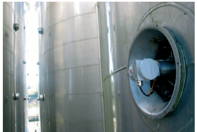
Figure 4: DT302S Installed on a Fermentation Tank
