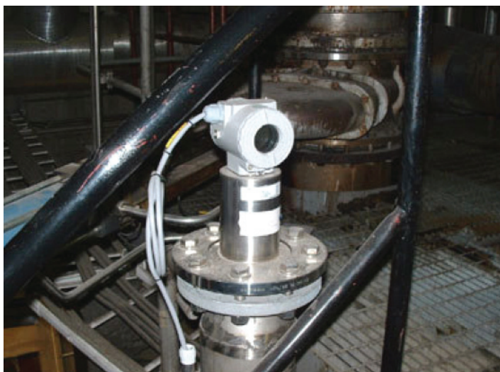
DT301 installed at Stora Enso-Sweden
